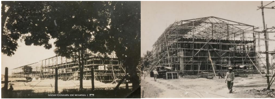
Figure 2 The Construction of the ASRI Building in 1957 (Source: Yogyakarta Nusantara Art Foundation)
