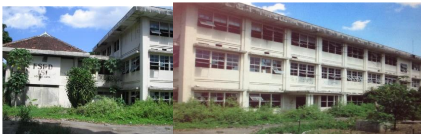
Figure 3 The ASRI Complex, which experienced damage in 2006 (Source: Jogja National Museum document )
