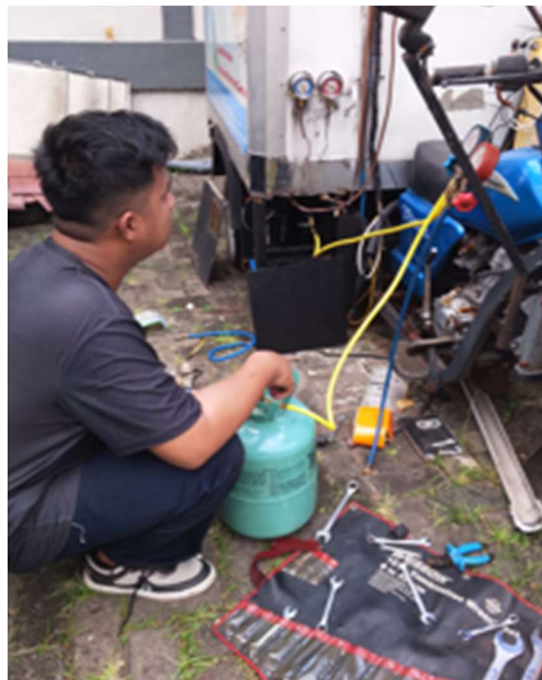
Figure 2 Testing and Filling of R22 Freon
